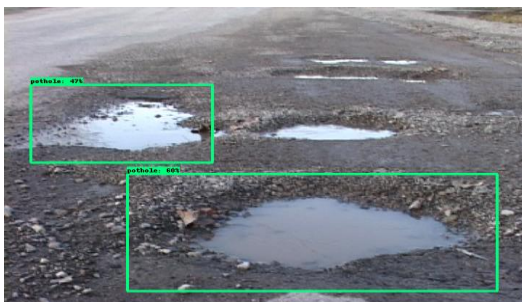
Figure 1: Potholes in roads
